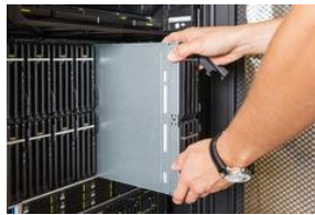
Data Center Blade Server
